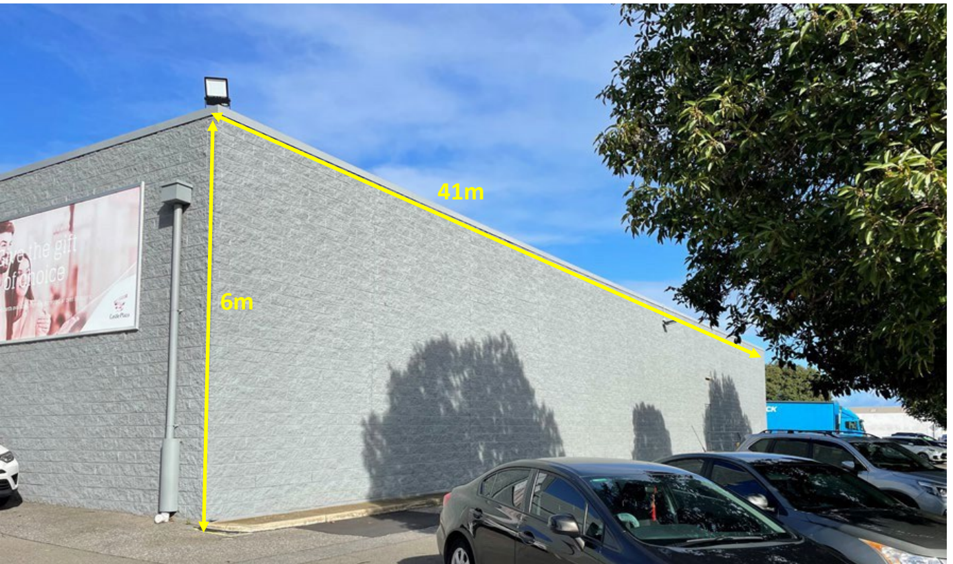
Castle Plaza Shopping Centre wall for 'Edwardstown: we're making it' messaging and branding, mural and approximate wall measurements
